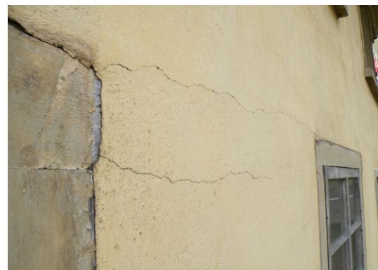
Fissures de joints
