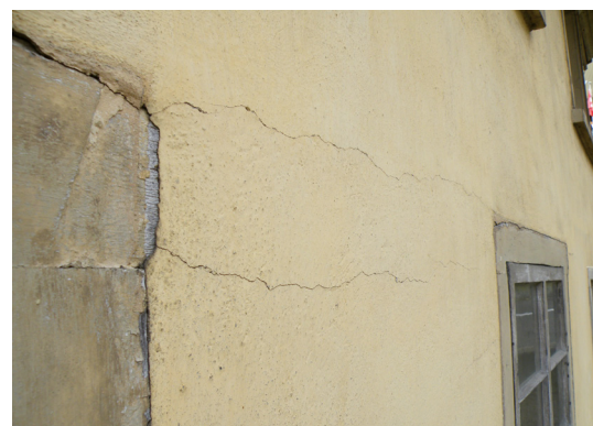
Fissures de joints
