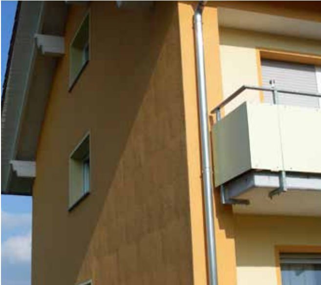
Facade of insulating panels illuminated in angled light. The outline of individual panels is visible under the surface but in accordance with SIA 243 «Rendered exterior thermal insulation» must be accepted as such.
