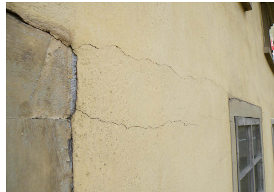
Fissures de joints
