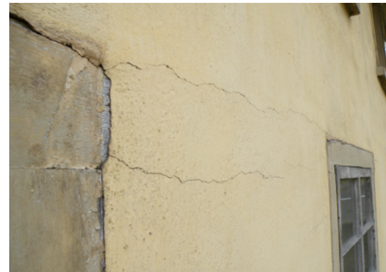
Fissures de joints
