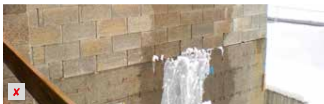
Vlažni tzv. mantelbeton
