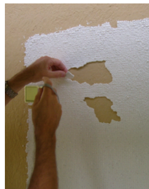
Support insuffisamment porteur
