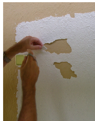
Support insuffisamment porteur
